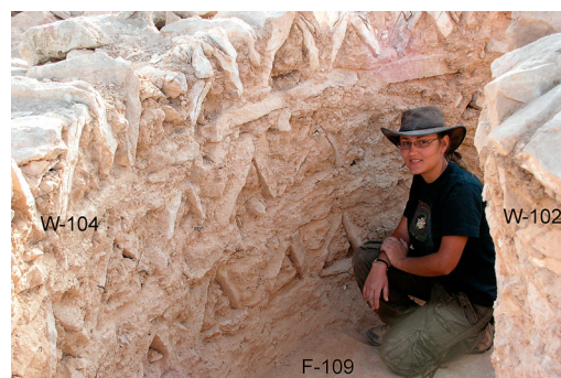
Figure 6 Structure A at Sa'adon with stone-built pigeon nests in the inner part of the peripheral wall (Photo: Yotam Tepper).
